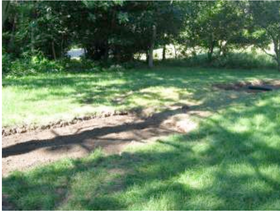
Mary Tilly Project – 2 of the 4 raingardens excavated on Mary Till Property. Perforated pipe from home downspouts directs runoff to raingardens and away from the St. Croix River.
